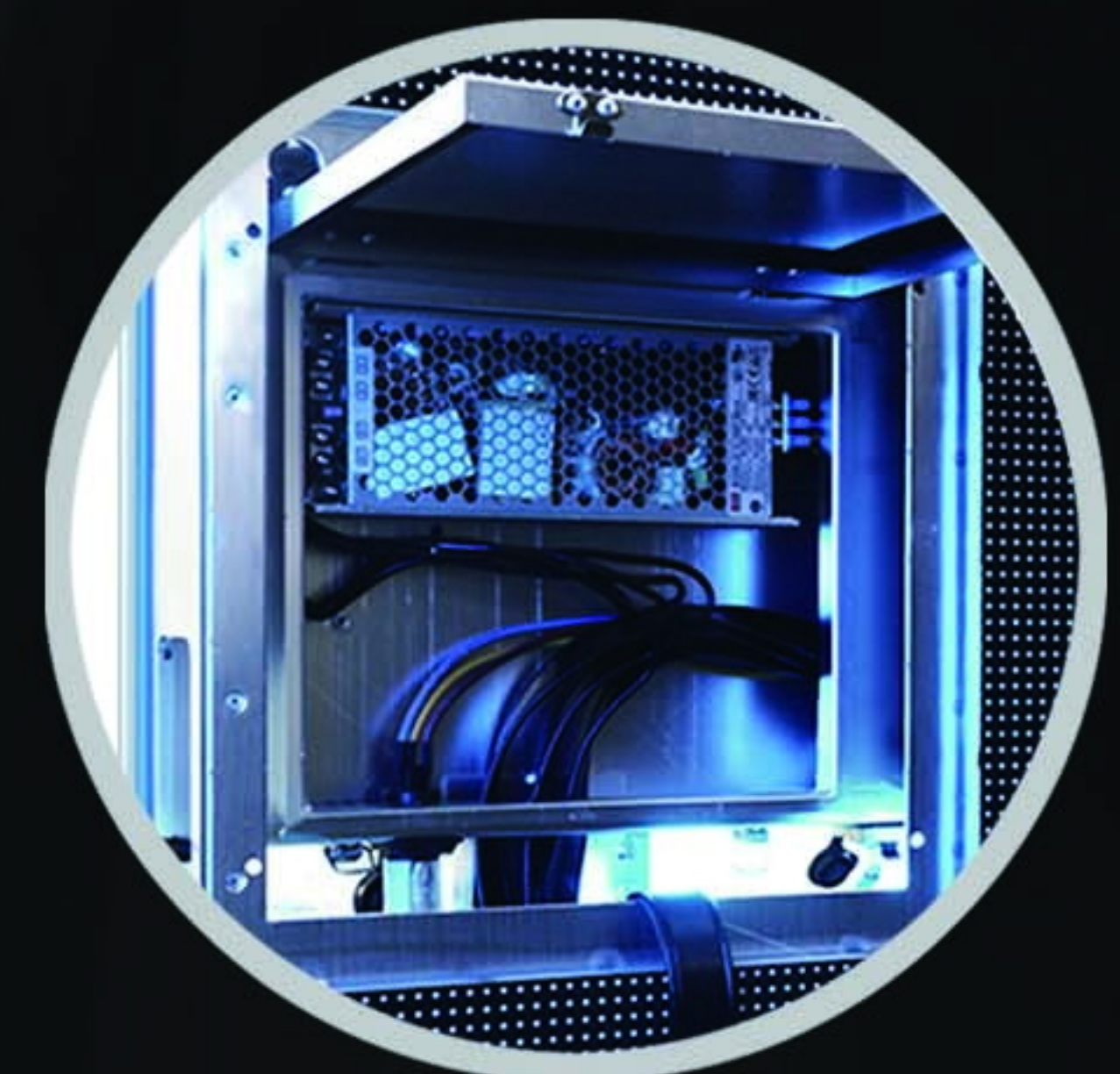
Power supply front and rear maintenance
